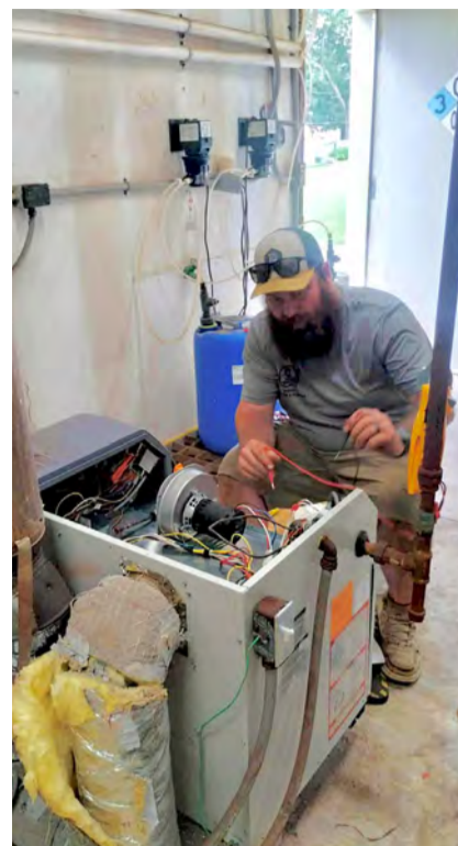
Murphy's Heating & Plumbing Co-Owner Keegan Murphy working on the pool heater on Thursday, Aug. 28.
