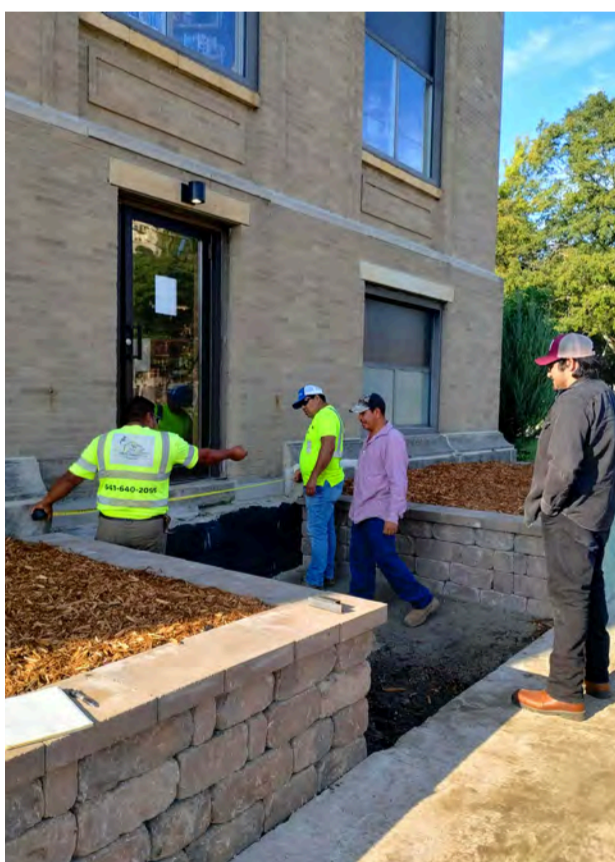
Tony's Concrete team and Max Alfaro checking out the space they have to work with on Friday morning.
