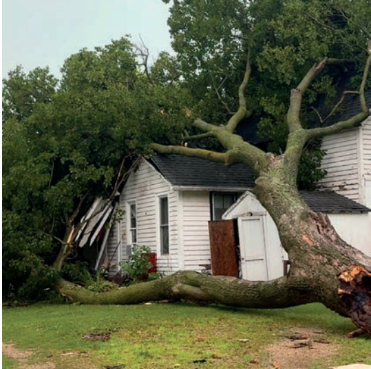
Kylee and Jessica Janssen's storm-damaged home after a large tree crashed through the roof during severe storms in Hampton.
