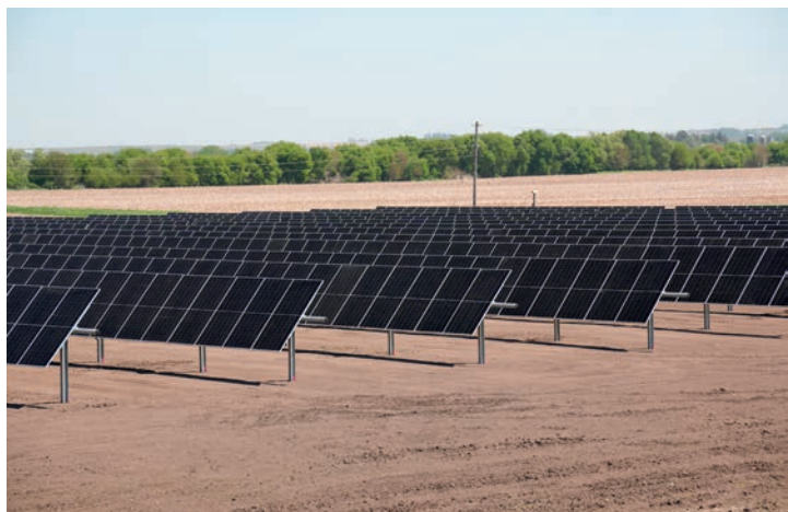
A view showcases Franklin General Hospital's solar array, which helps provide renewable energy to support the hospital's daily operations.
